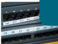
Punch block & patch panel labels
